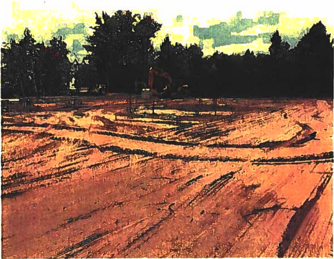
Looking South from site entrance: Common excavation and fill completed, select fill installed and compacted for drive and parking, building foundation and slab installed.
