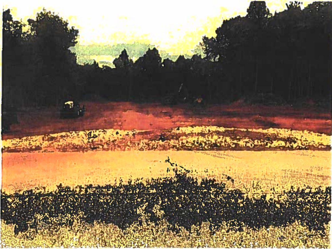
Looking South from site entrance: Site cleared and grubbed and stabilized construction entrance installed.
