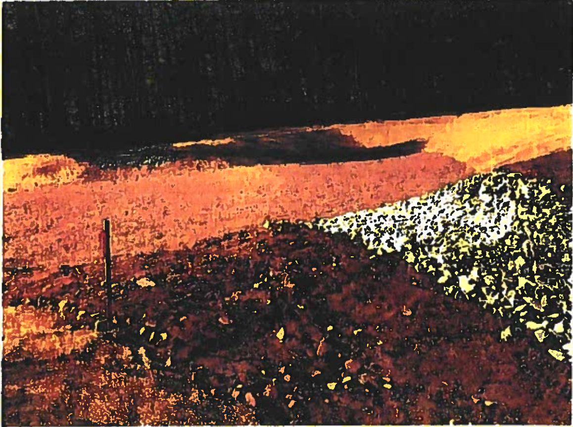
Looking South from outlet of forebay: Filter medial installed and consolidated, stone outlet protection for both forebay and infiltration basin installed, loam seeded and mulched.
