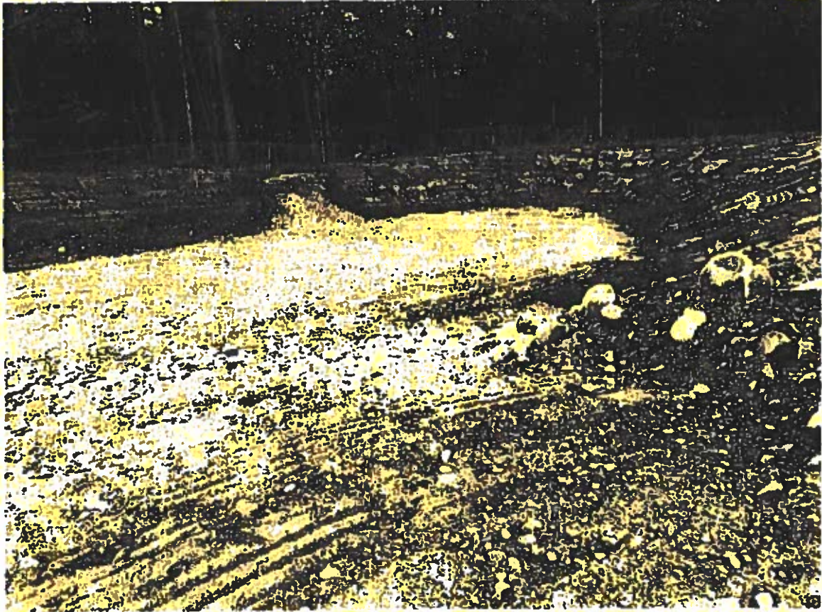
Looking South from outlet of forebay: Native soil under infiltration basin scarified before installing 24 inch thick filter medial. Installation of loam limited to side slopes of infiltration basin.
