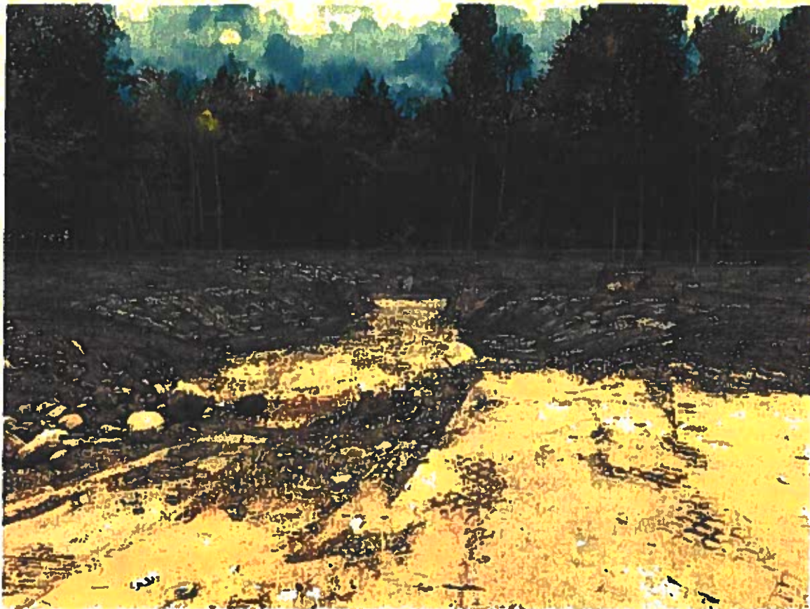
Looking South near end of paved parking: Common excavation and fill completed for forebay and infiltration basin, Loaming completed for side slopes for forebay, infiltration basin, and adjacent grassed areas.
